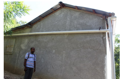
Above: Gutters on Savannah School - Oct. 3, 2020
